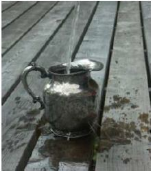
Corrosion Pits are the primary source of leaks in water handling systems
