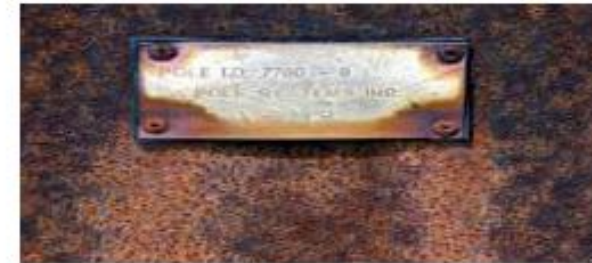
Galvanic corrosion between Steel and Brass.
